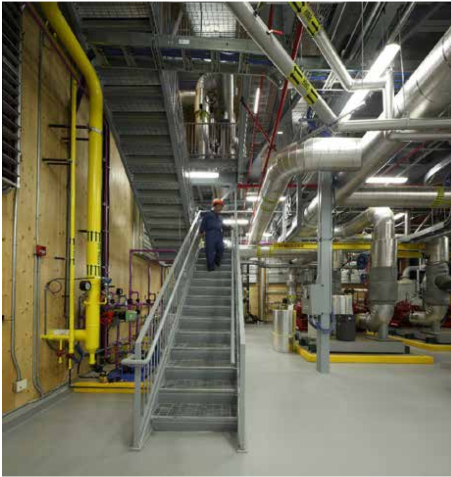
Photo 5 – Interior View of Equipment
