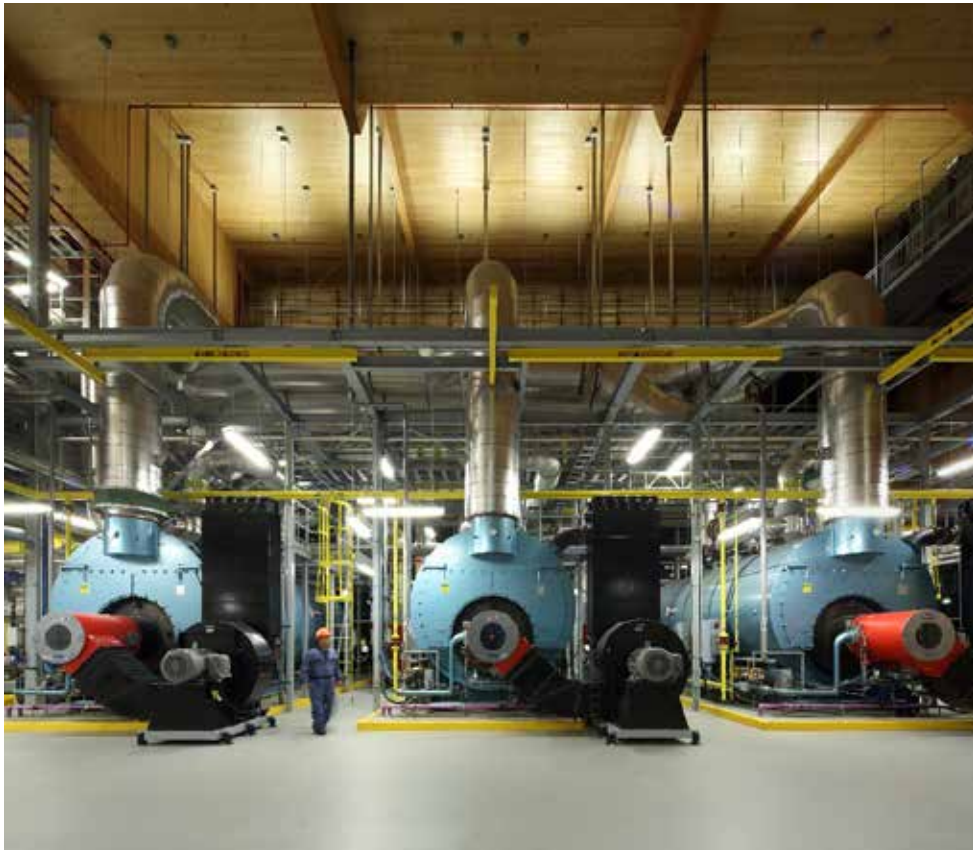
Photo 3 – Interior View of Equipment
