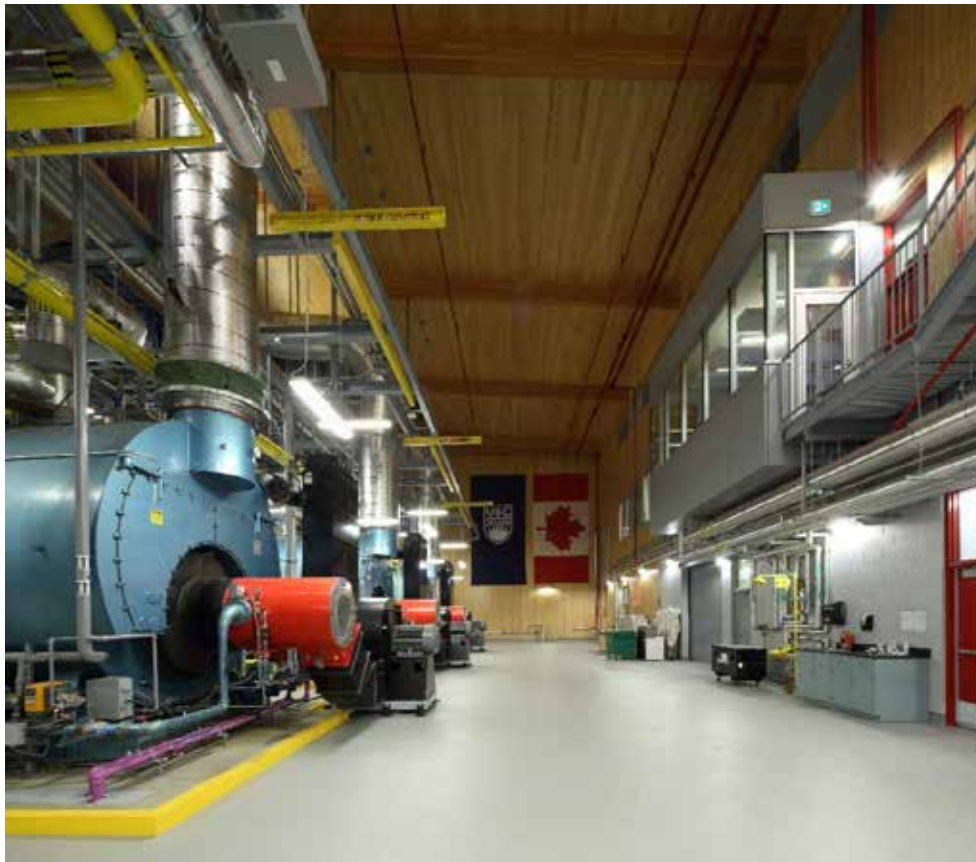
Photo 4 – Interior View of Equipment
